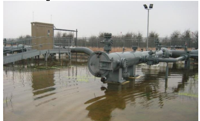
Figure 22.19 flooding at the Gravesend Thames South above ground installation in 2013
